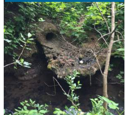
Stormwater outfall into Glenn Creek currently about 12" above the existing streambed
